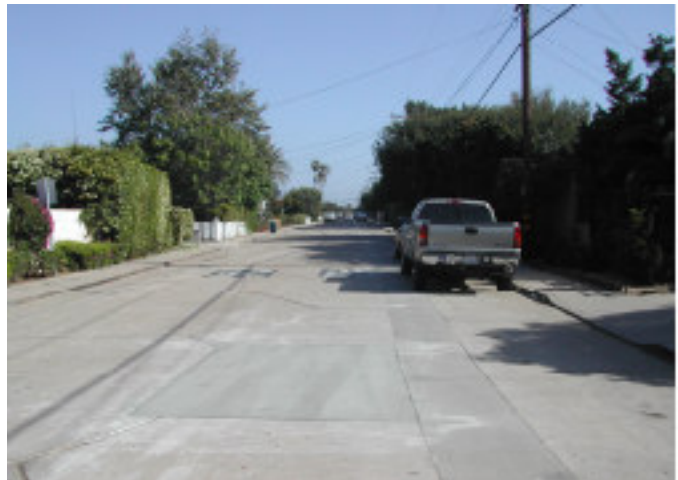
Pacific Avenue is a local road that has curb, gutter and sidewalk.
