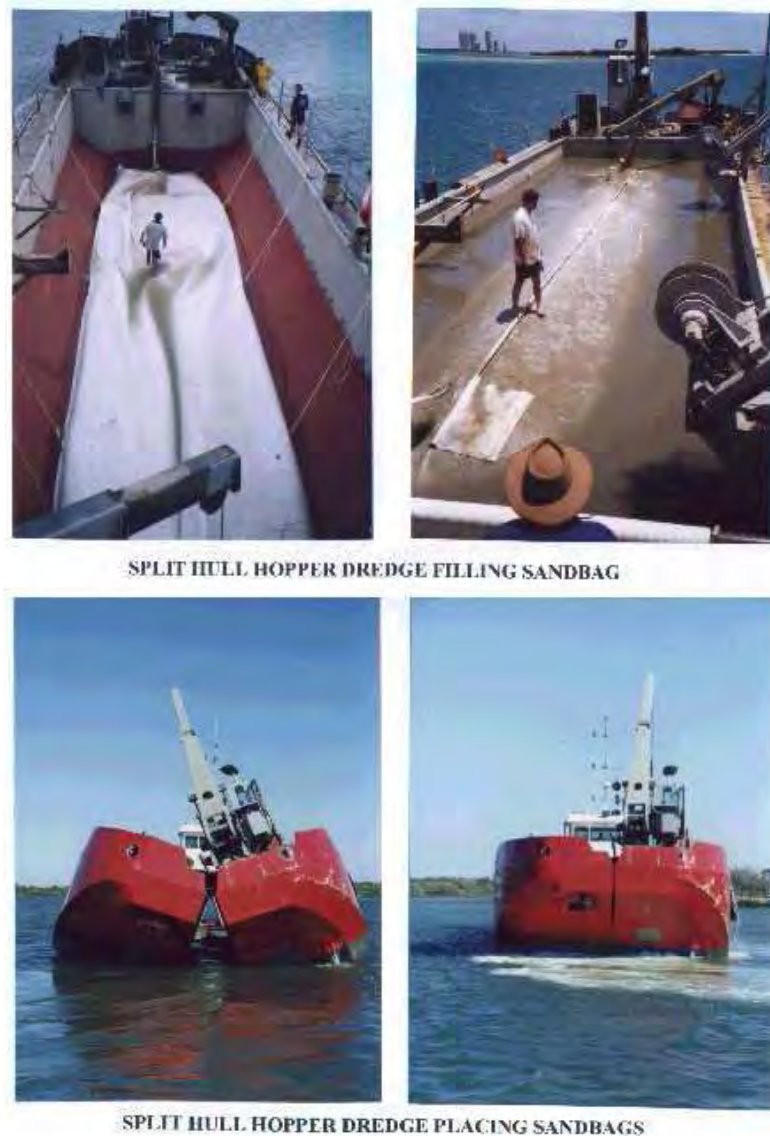
Figure 2. Terrafix 1200R SFC's being filled and placed during construction of the Gold Coast reef.
