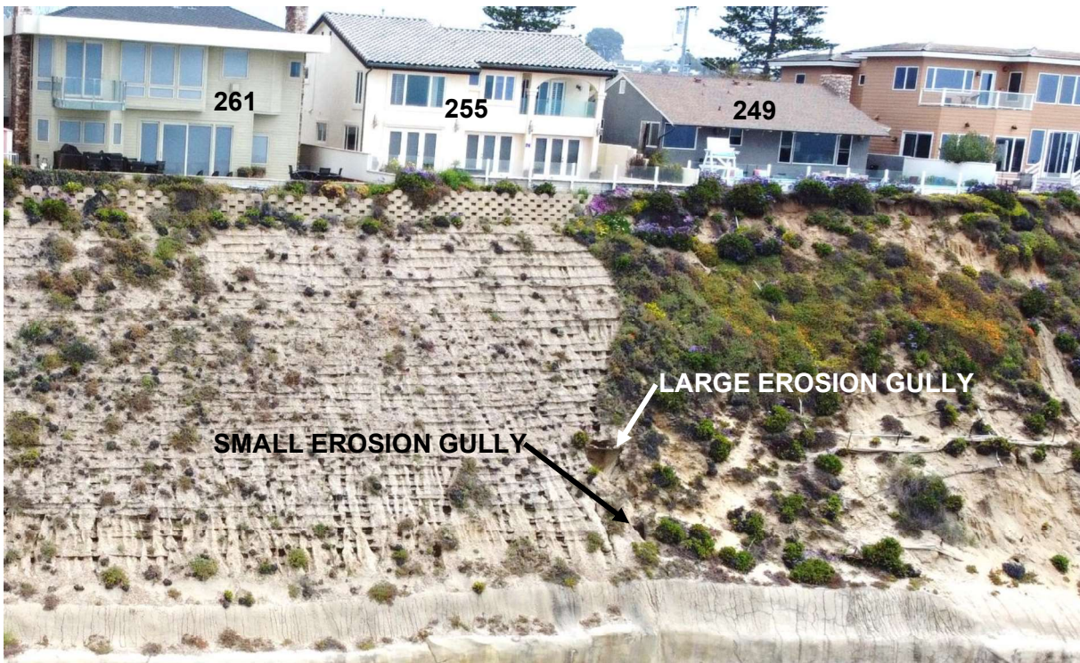
Photo 13: Geogrid-reinforced slope below 261 to 249 showing signs of deep erosion (April 26, 2023).
