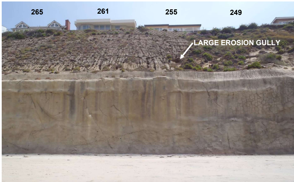
Photo 12: Upper bluff below 265 to 249 Pacific Avenue (April 26, 2023). Geogrid-reinforced slope is showing continued rill erosion due in part to lack of vegetative cover.
